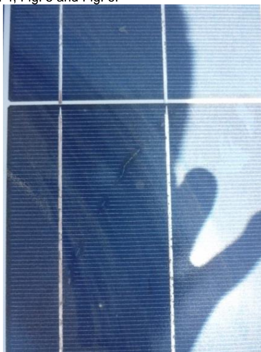
Fig. 4: Snail trail founded in the PV-system (a). Source: sent by the installer, taken in situ
