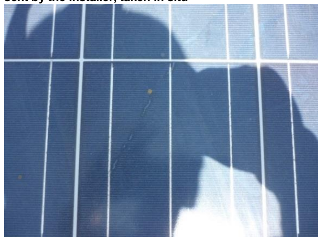
Fig. 6: Snail trail founded in the PV-system (c). Source: Pictures taken in situ
