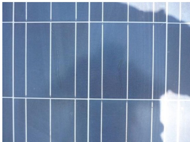
Fig. 5: Snail trail founded in the PV-system (b). Source: sent by the installer, taken in situ
